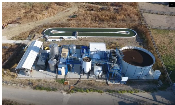
Fig. 16: Water2REturn system at Matadero del Sur
