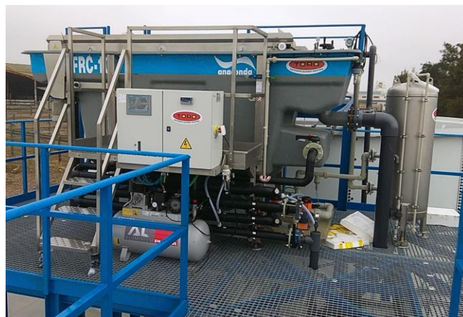
Fig. 9: Water2REturn DAF unit
