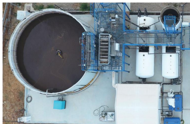
Fig. 4: Water2REturn water line
