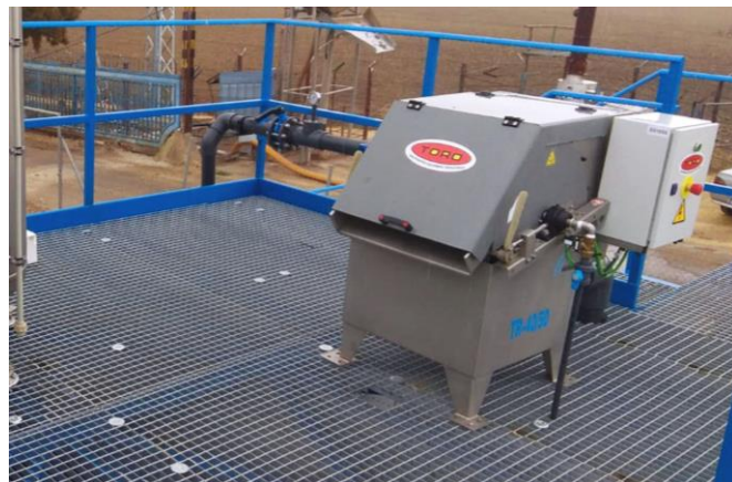
Fig. 8: Water2REturn solids separation unit (rotary screen)
