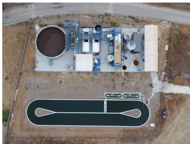
Fig. 15: Water2REturn system at Matadero del Sur
