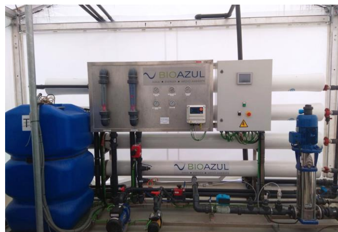
Fig. 14: Water2REturn reverse osmosis
