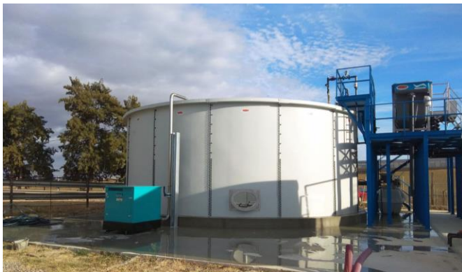
Fig. 11: SBR de Water2REturn
